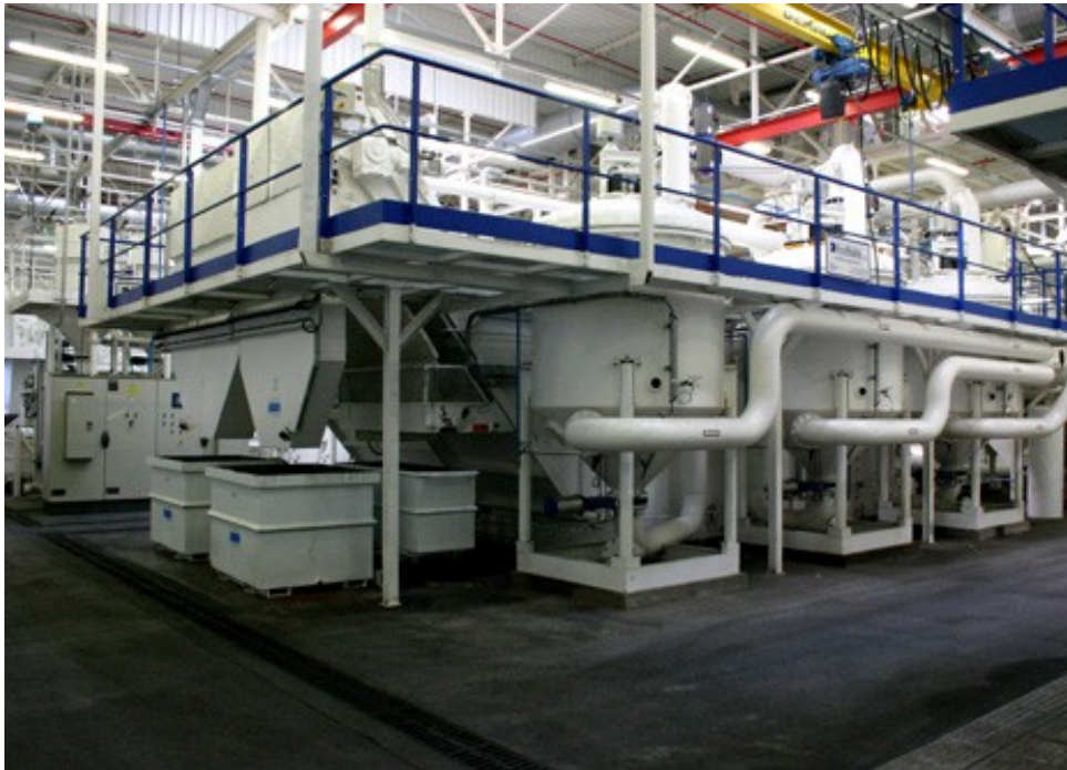
Filtration unit for 600m 3 /h grinding at PSA (2003) - Flex
