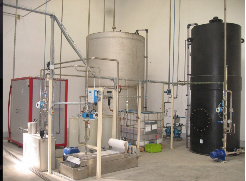
Effluent treatment by evaporator (Dacia Romania 2007)
