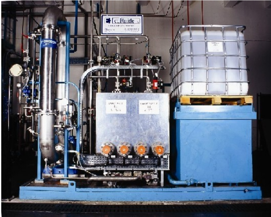
Ultrafiltration unit (FM)
