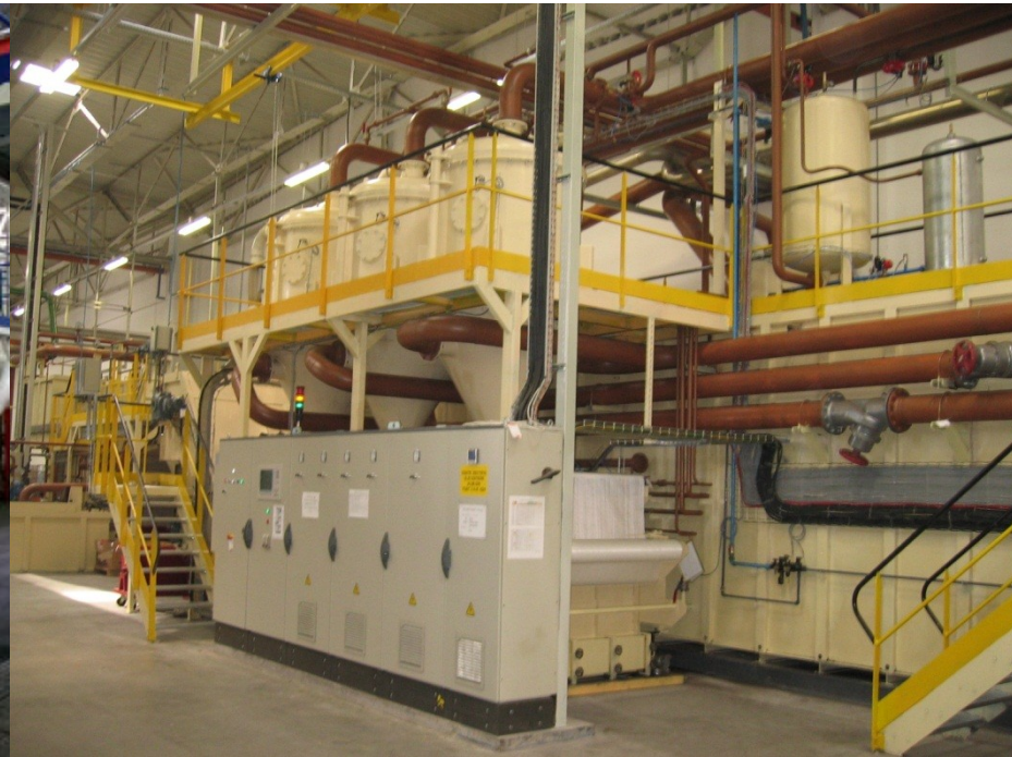
Filtration unit for 300m 3 /h grinding at Dacia (2007) - Candles
