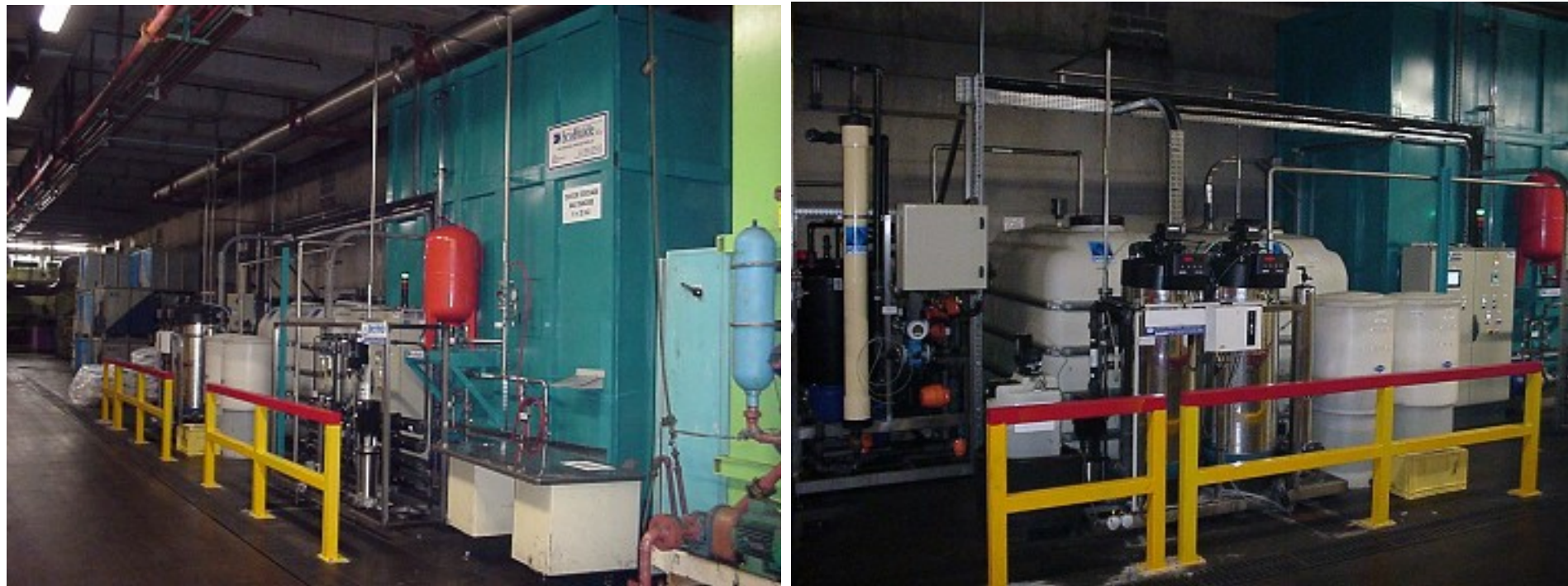
Osmosis unit (FM)
