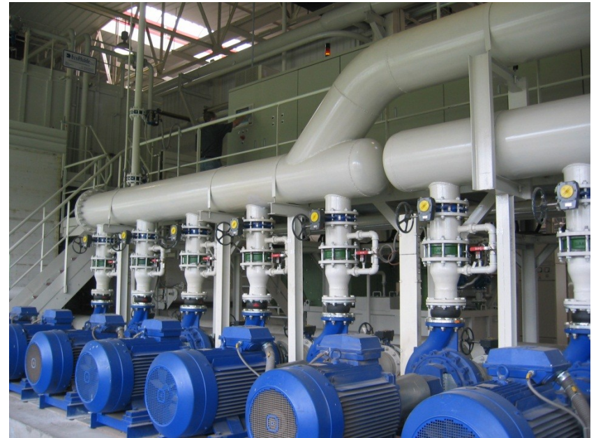
➤ The Supplying Pumps Group: 10 Pumps x 90 kW/pump
